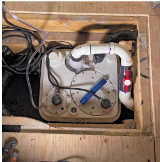
The Sanicubic 1 positioned in a small space under the floating home’s wooden floorboard. AR Plumbing owner and CEO Adello Rodas and his team used two of the four inlets on the Sanicubic 1.
