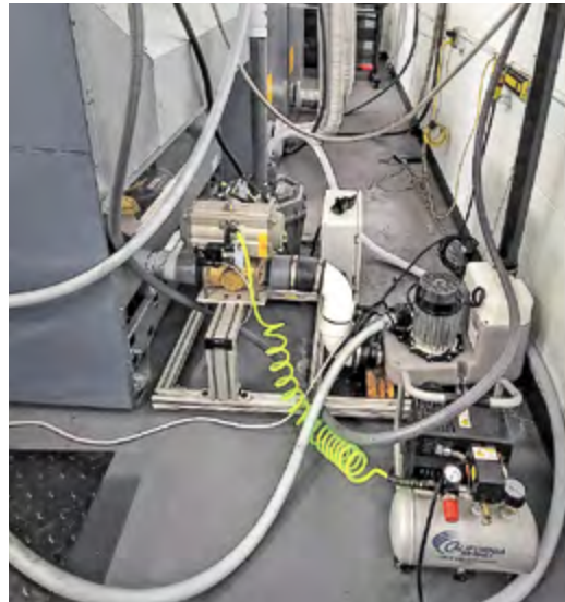
The pretreat coming from the washing machines flows into the Sanicom unit. The Sanicom pumps the liquid five feet via hose into the reuse tank connected to the washing machine.
