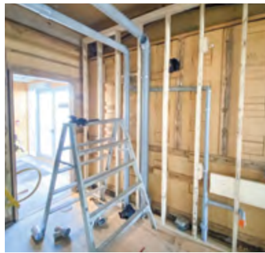
The drain lines coming from the washroom loads and the load from seven hotel suites running to the Sanicubic 2VX.
