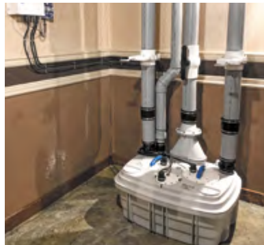
Albanese installed the Sanicubic 2VX in the hotel's basement. The 4-inch discharge pipe runs from the top of the Sanicubic 2VX 10.5 feet vertically and 25 feet horizontally before tying into the existing drain line.
