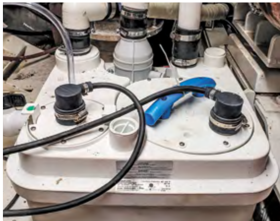
Inside the RV MANTA's mechanical room, showing the Sanicubic 1 and the 1.5-inch PVC piping to two of the Sanicubic 1 's four input ports.
